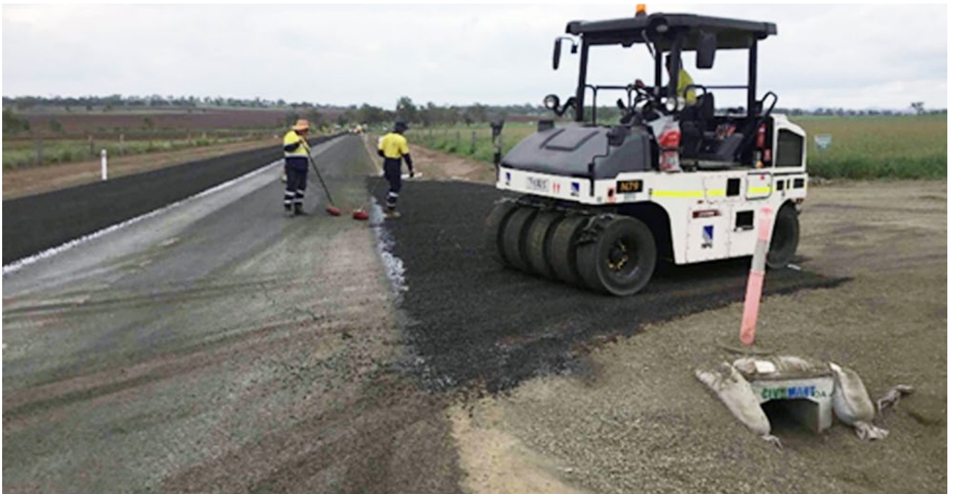
Bowenville Moola Road – multiple coat treatment on private accesses to withstand load from trucks
